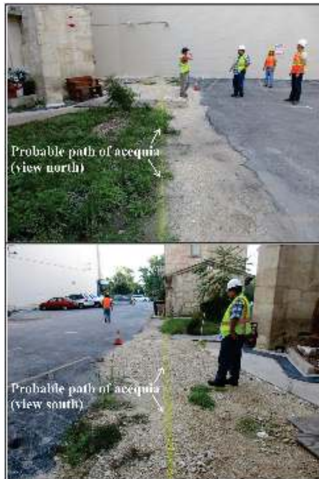
Figure 4-1. Plotting the probable path of the acequia with marking paint, north of the Rectory.
