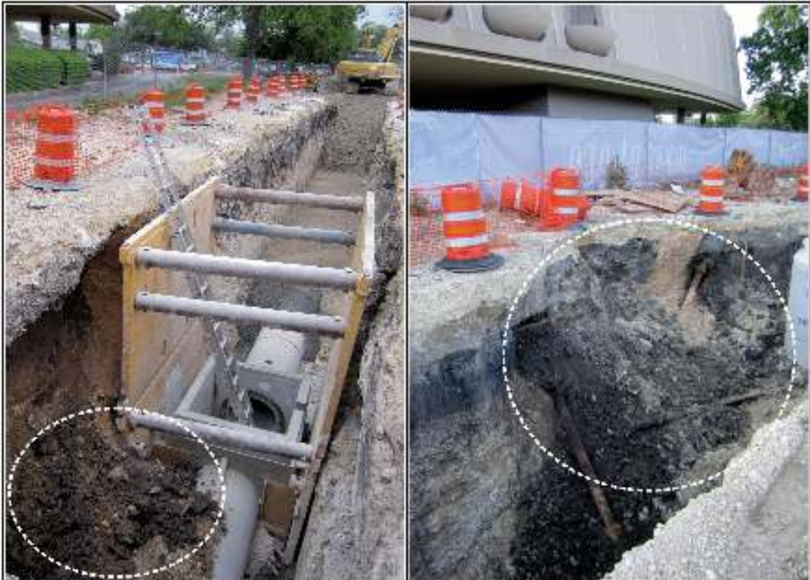
Figure 8-7. Typical wall collapse of storm drain trench on Hemisfair Way, view south (right), and storm drain trench on Hemisfair Way (view southeast) to the immediate west of Adrian Spears Judicial Training Center (left).
