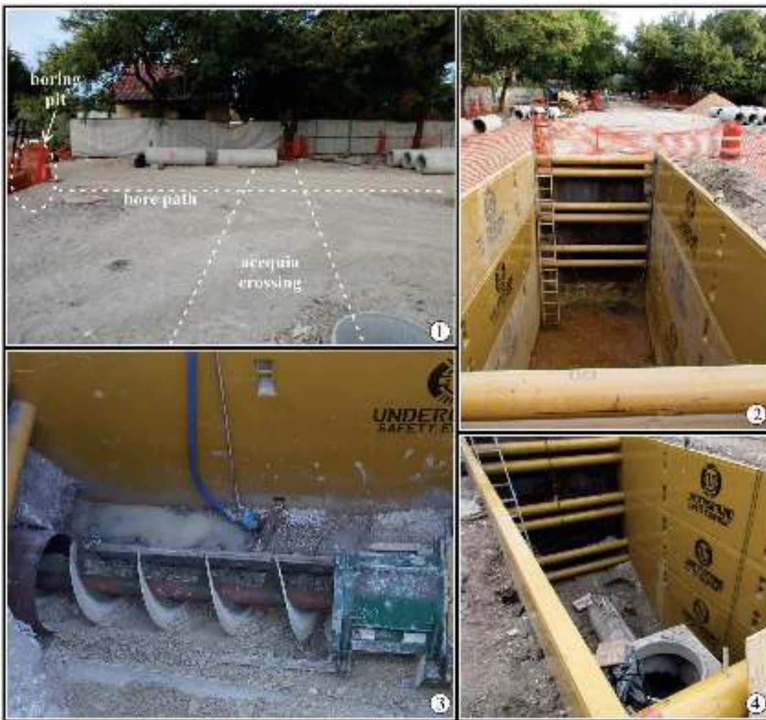
Figure 8-8. Boring process to install storm drain underneath Acequia Madre de Valero (41BX8): 1) acequia crossing, facing south; 2) boring pit, facing west; 3) boring and steel casing installation in progress, facing north; and 4) storm drain installation in progress, facing northwest.
