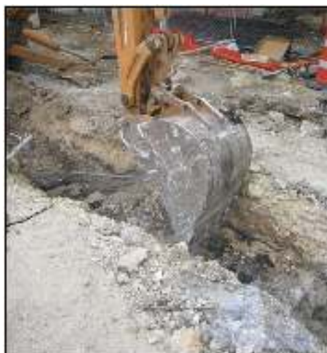
Figure 8-20. Water line trenching along E. Nueva Street, west of the acequia crossing (facing southeast).
