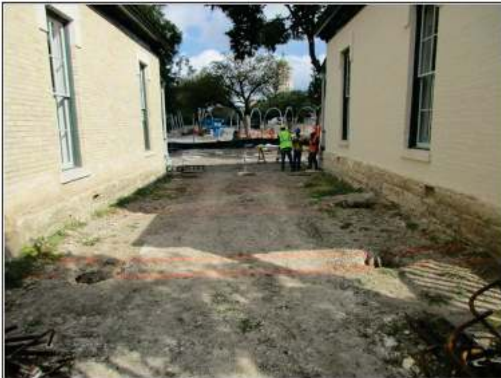
Figure 7-8. Four trenches excavated between the Koehler (41BX592) and Espinoza (41BX593) houses (facing east).
