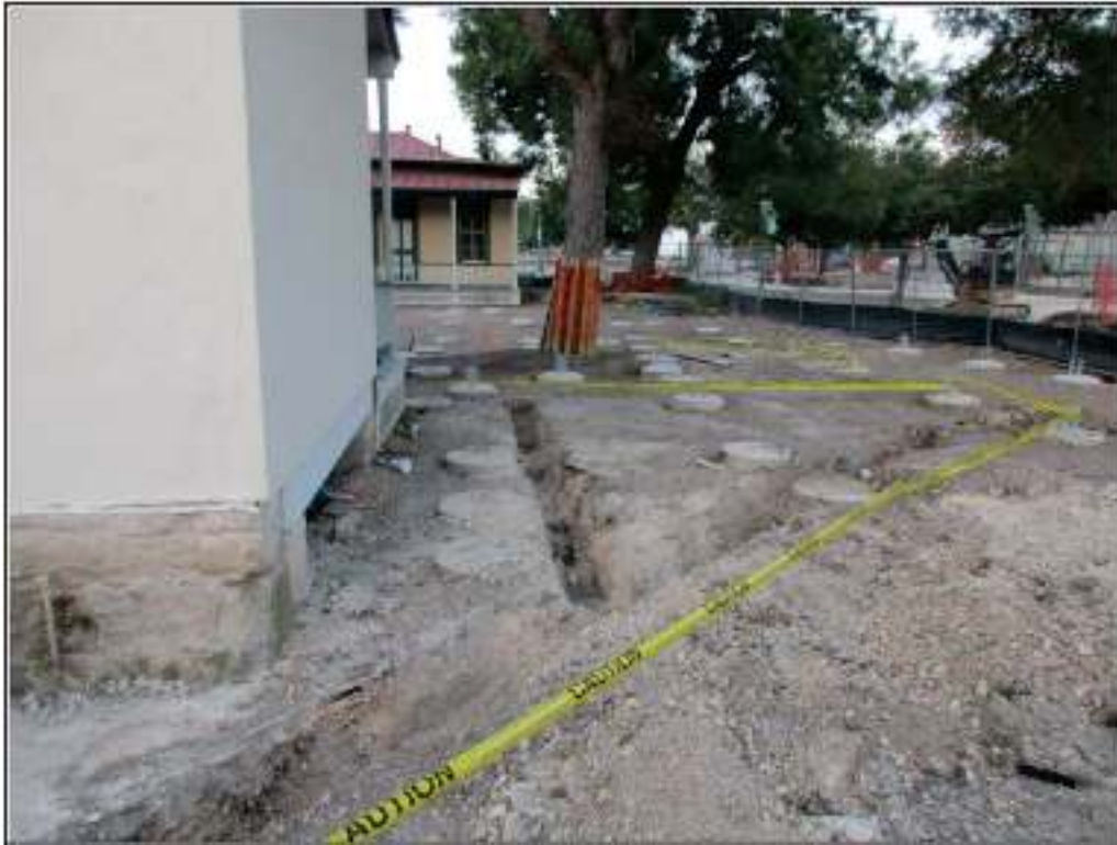
Figure 7-10. Trenches excavated for water lines to service the Koehler House (41BX592) and the Espinoza House (41BX593), facing south.
