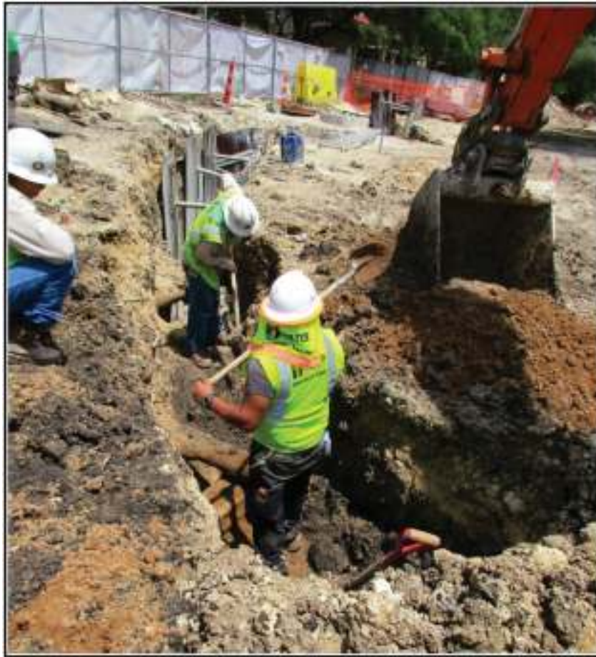
Figure 8-13. Duct bank work along west end of E. Nueva Street (facing east); note the need for hand excavation due to the utility crossing.
