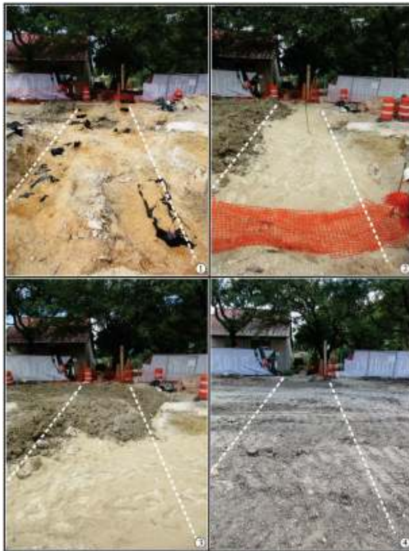
Figure 8-25. Acequia Madre de Valero (41BX8), backfilling stages: 1) landscape fabric and sand covering acequia walls; 2) additional layer of sand; 3) layer of clay fill; and 4) covering completed.
