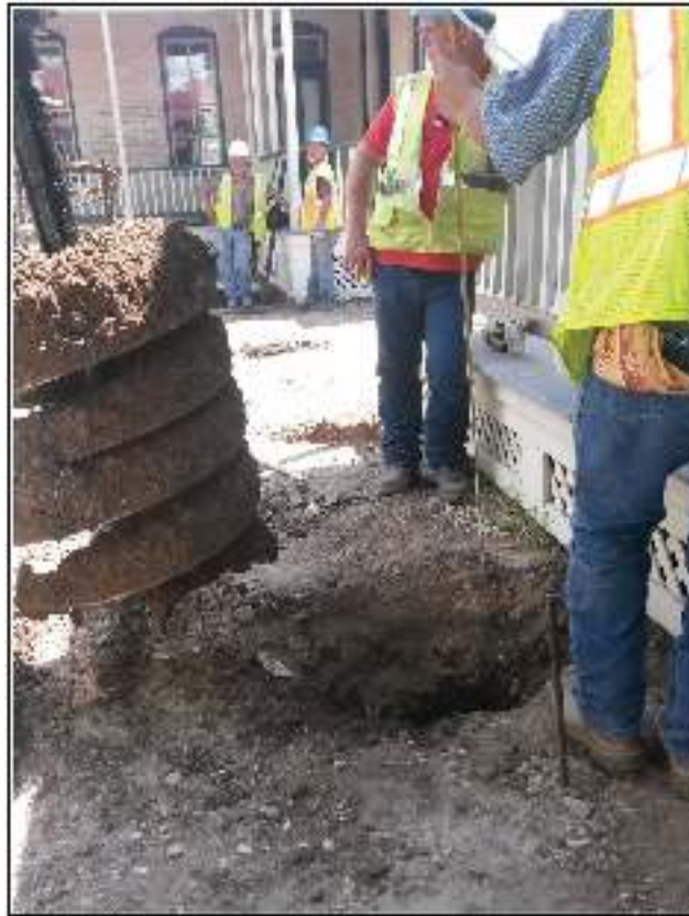
Figure 7-7. Spot monitoring the excavation of piers at the Koehler (41BX592) and Espinoza (41BX593) houses.
