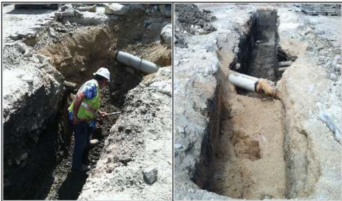
Figure 8-30. Gas line install, north side of E. Nueva Street at acequia crossing; note area is heavily impacted.
