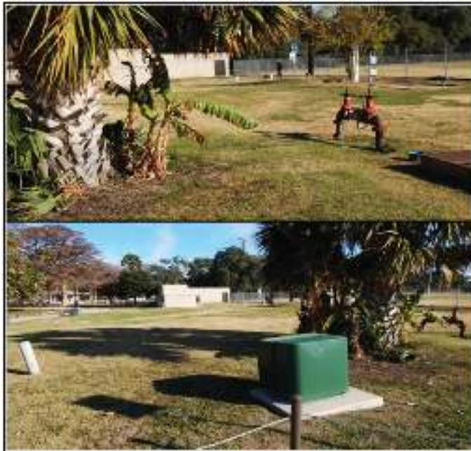
Figure 9-6. Additional utility lines associated with area of acequia. Building in top and bottom photos is visible in Figure 9-5 to right.
