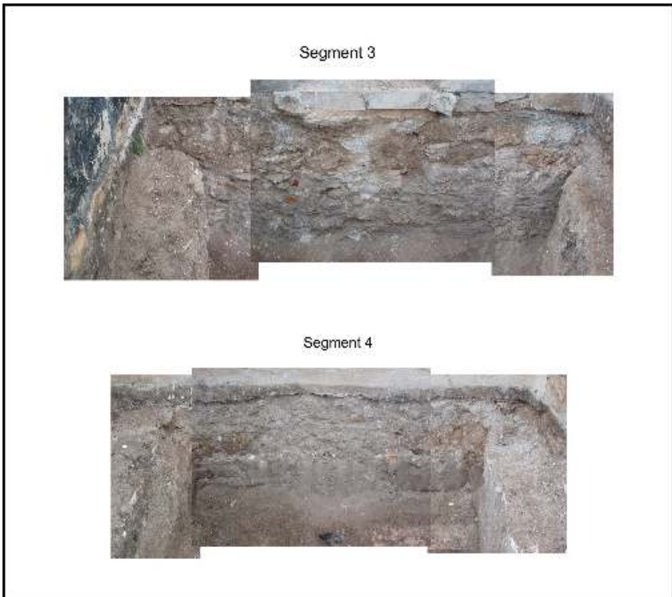
Figure A3-2. Segments 3 and 4 of the foundation of the east wall of the church, middle portion.
