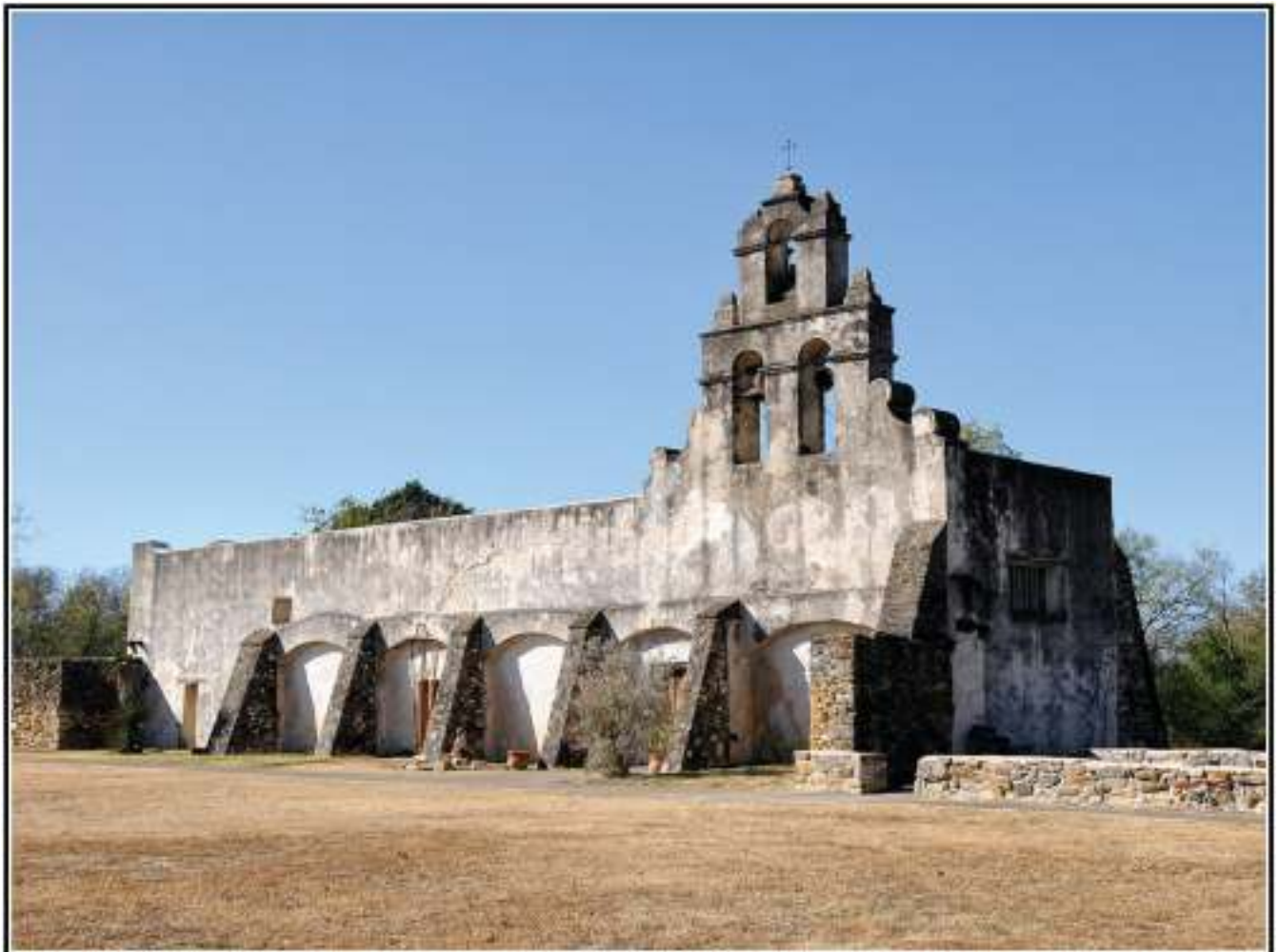
Figure 1-1. The Church at Mission San Juan prior to the initiation of the underpinning.
