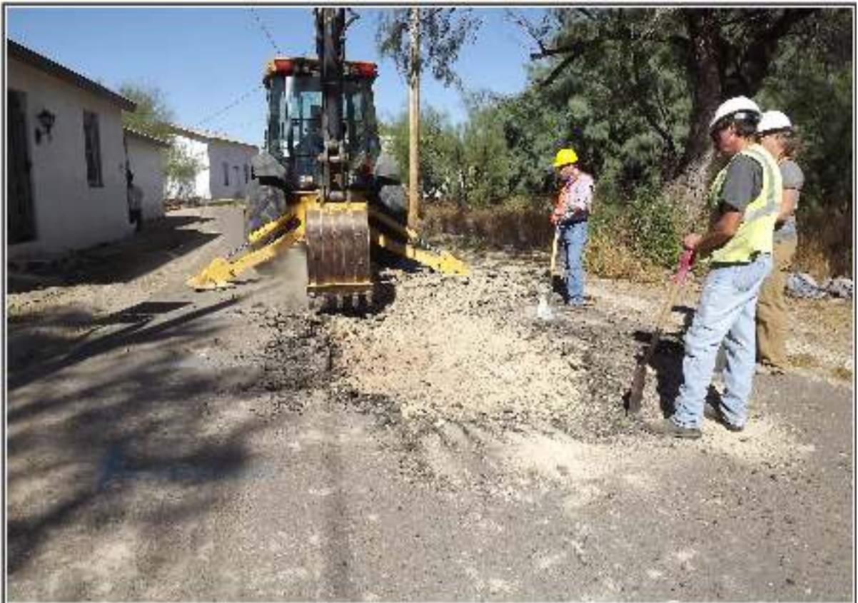
Figure 3-1. CAR archaeologists monitoring the mechanical removal of the pavement over the burial.
