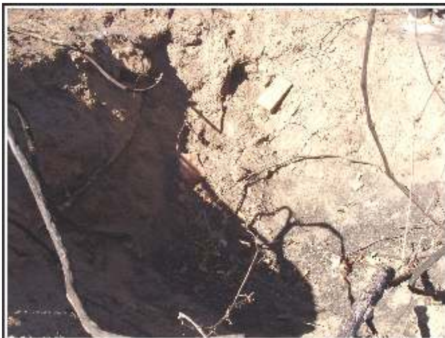
Figure 5-9. Collapsed well on previously recorded historic site 41BP430.
