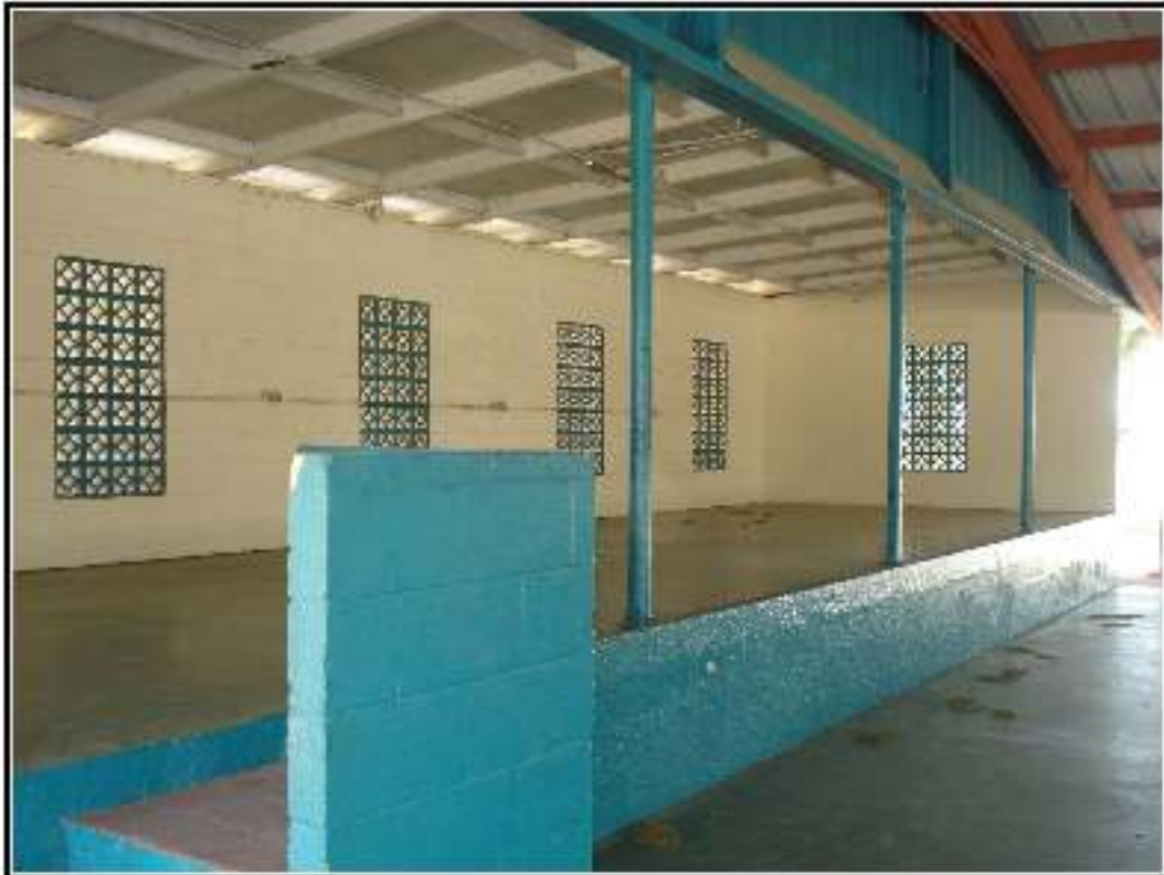
Figure 5-12. Stage-like feature along one side of structure 2. Note decorative window details in concrete block wall.
