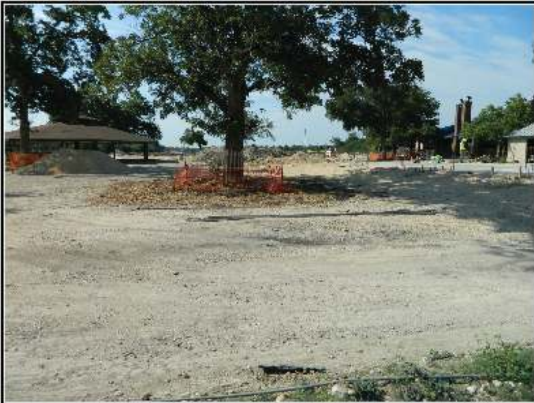
Figure 5-22. Administrative complex after the demolition of the targeted structures. Note structures 1 and 5 in the mid-ground.
