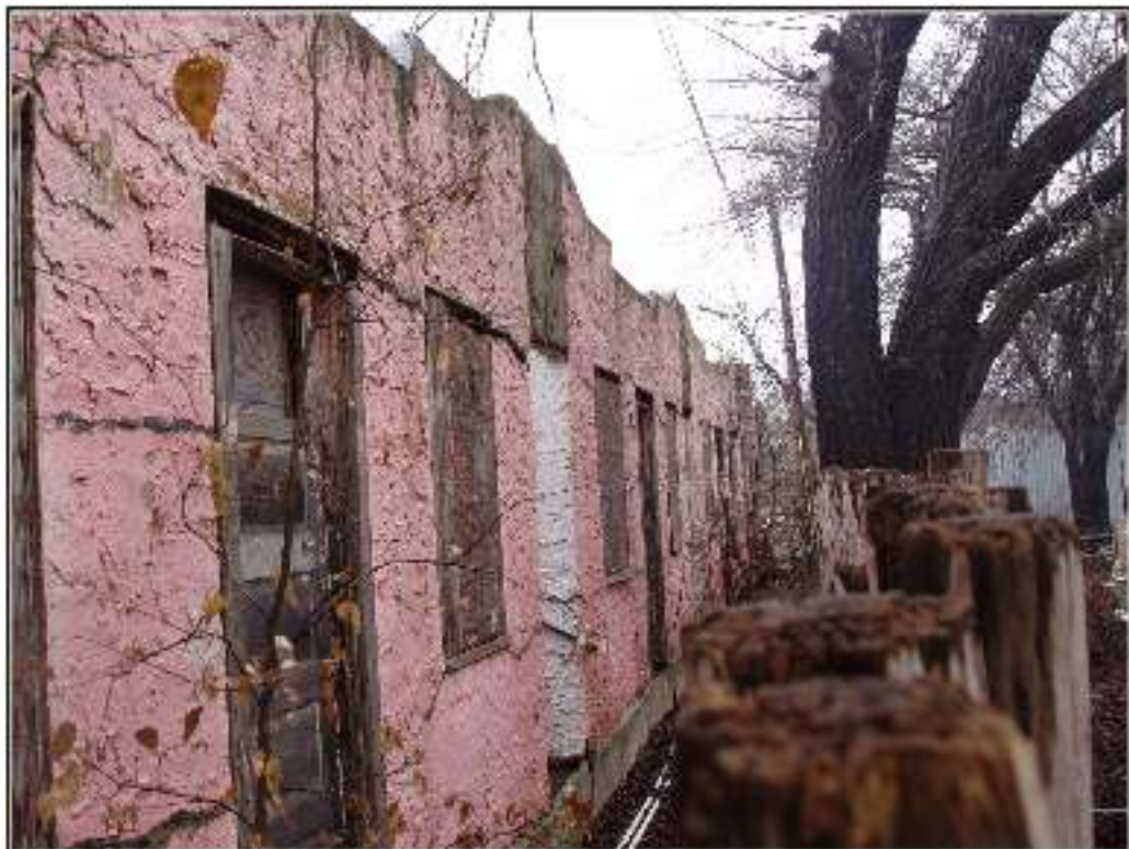
Figure C-27. The single story guest houses of the historic Kimble Courts have been demolished but are illustrated here in Spring 2005 in Junction, Texas, after they were moved in 1935 from the banks of the South Llano River.
