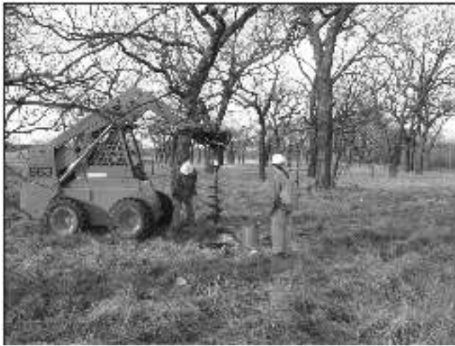
Figure 4-3. Bobcat mounted auger reached depths up to 120 cmbs during Phase II testing.
