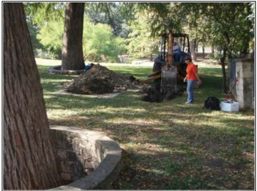
Figure 5-9. Excavation of BHT 5 just south of the Reptile Garden in the vicinity of the cypress trees. View toward the west.
