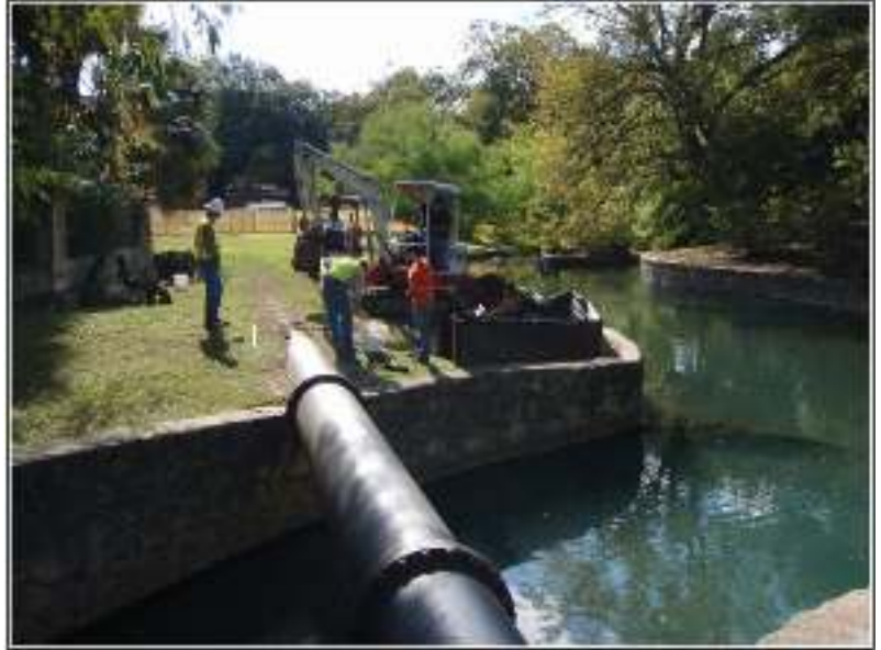
Figure 5-1. Excavation of BHT 1 near the stone-lined culvert (foreground) in the area between the San Antonio River and a 36" storm-sewer pipeline. View toward the south.
