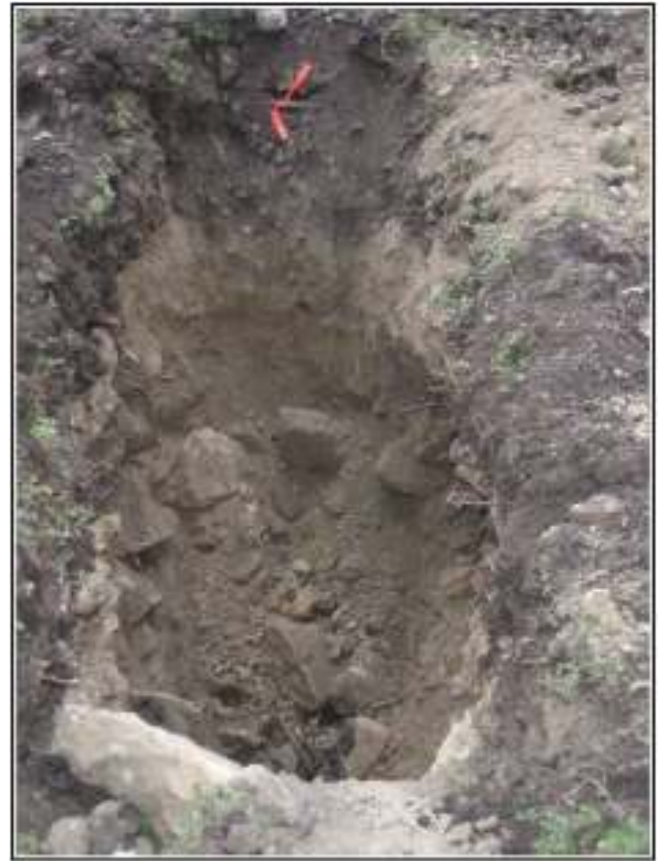
Figure 5-6. Unconsolidated fill materials encountered in BHT 3. Note the water pipe flagged with orange ribbon that caused the trench excavation to be abandoned. View toward the west.
