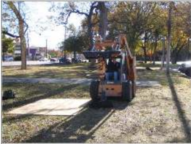
Figure 5-20. Excavation of Auger Boring 3 just north of the sidewalk leading to Pioneer Hall.
