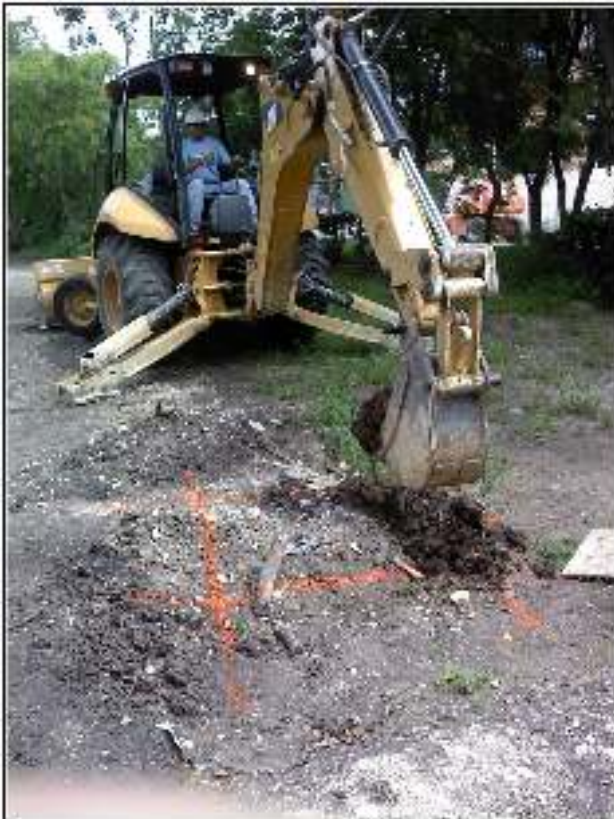
Figure 7-2. Backhoe excavating trenches for the installation of light posts along the hike and bike trail.
