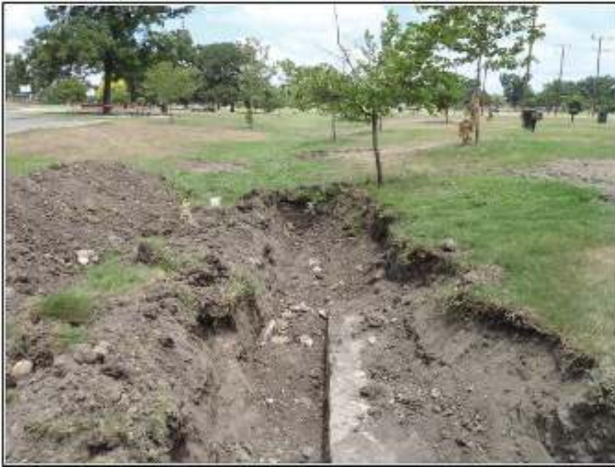
Figure 5-12. Edge of the stone wall near BHT 31 where it appears to have been disturbed.
