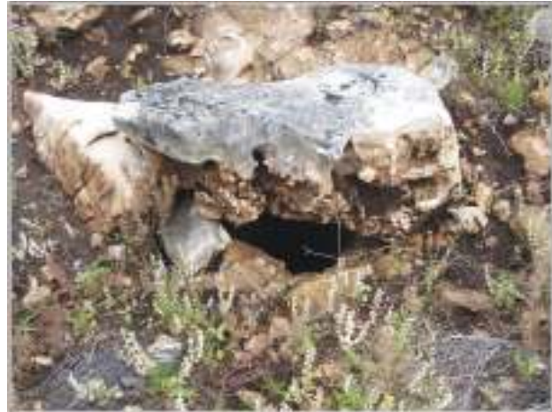
Figure 4-8. Sinkhole located near eastern boundary of the project area (note that the diameter is .3 meters).
