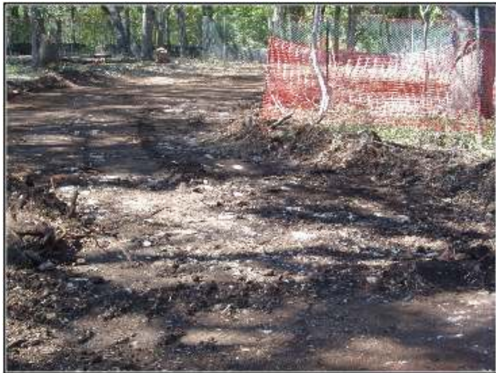
Figure 5-38. Bedrock exposed by the grading of topsoil across 41KE218. Edge of upland is at foreground where silt fencing is located.
