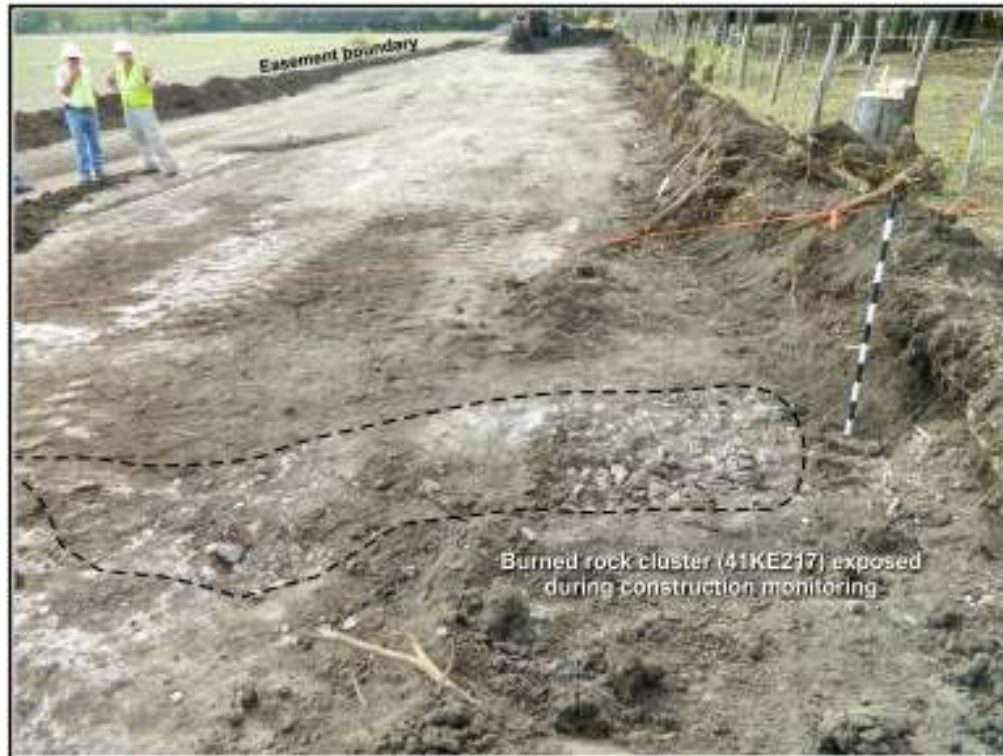
Figure 5-30. Overview of site 41KE217 during the initial discovery of burned rock zone, during construction monitoring. Facing south.
