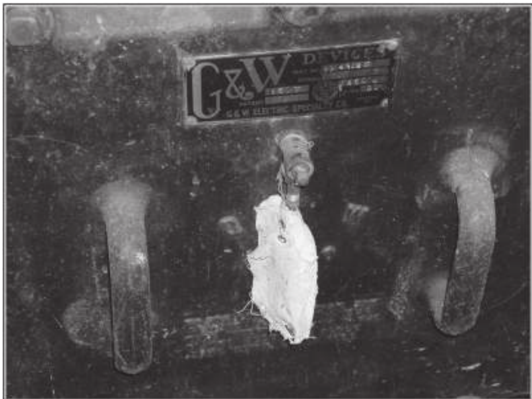
Figure 5-10. Front of the electrical cable junction box.
