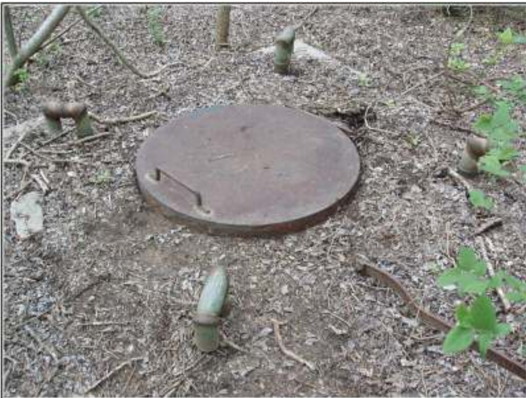
Figure 5-8. Electrical manhole located in the central portion of 41GD145 (see Figure 5-3).
