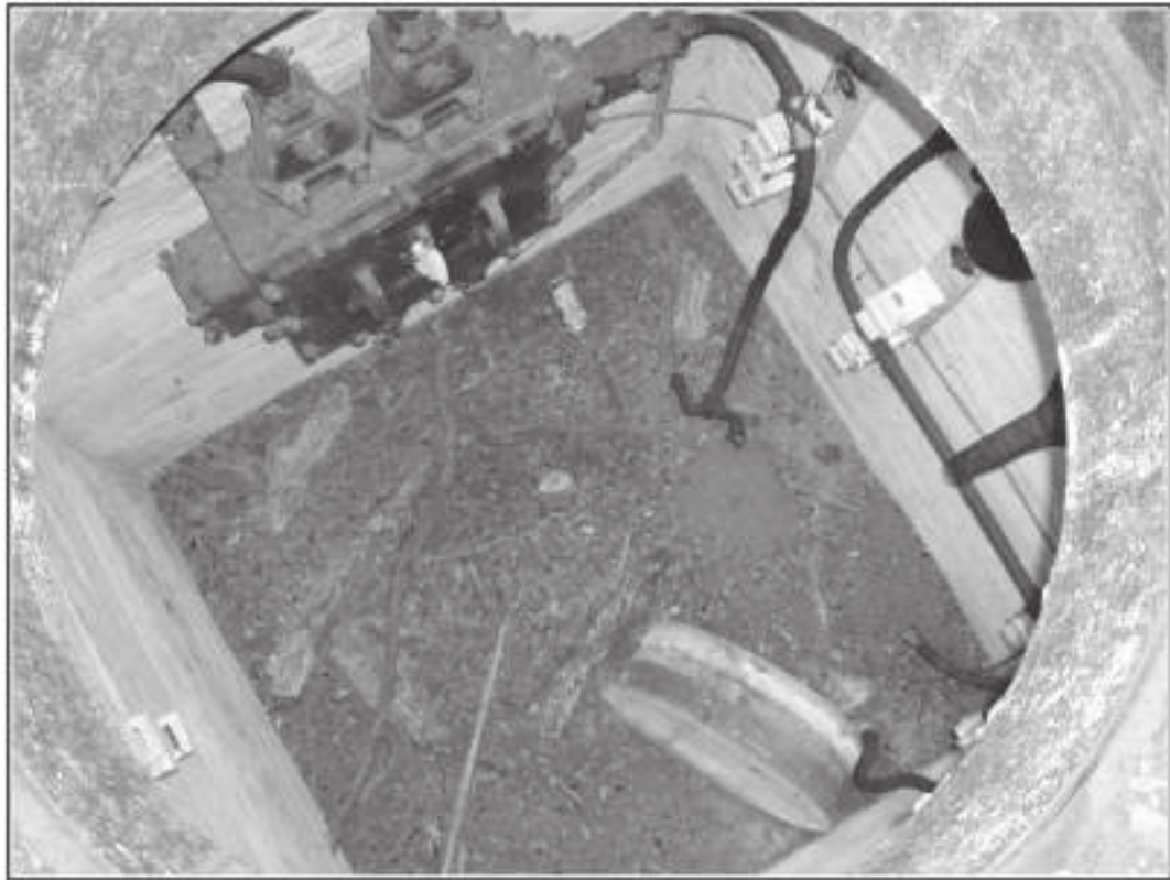
Figure 5-9. Inside of manhole showing the electrical cable junction box (41GD145).
