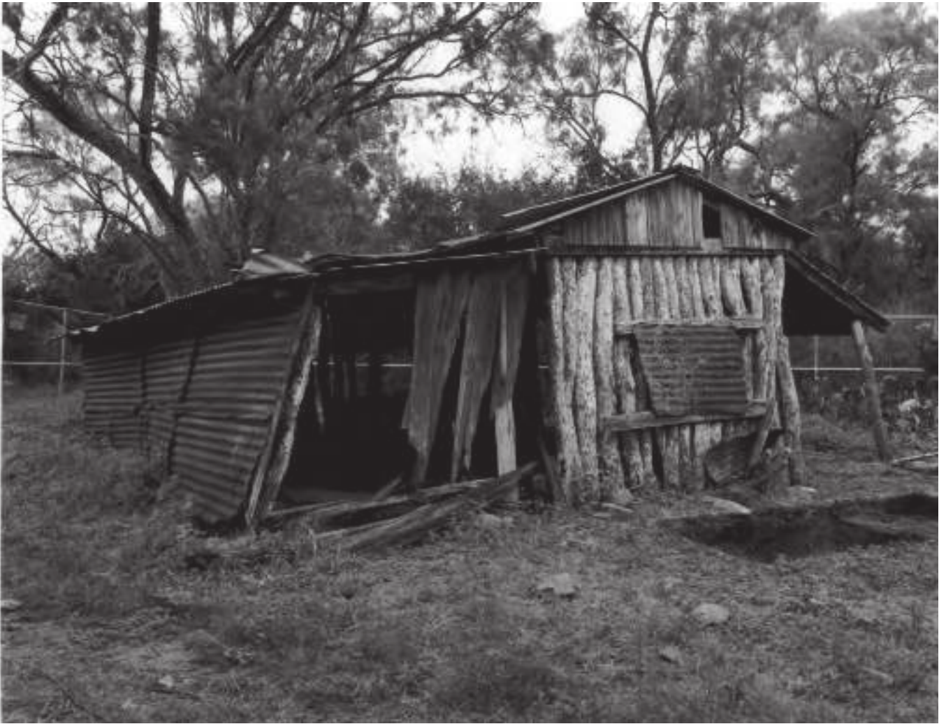
Figure C-9. View of jacal showing commercial and historic construction materials and damage, looking southeast (TX-3539-A-7).
