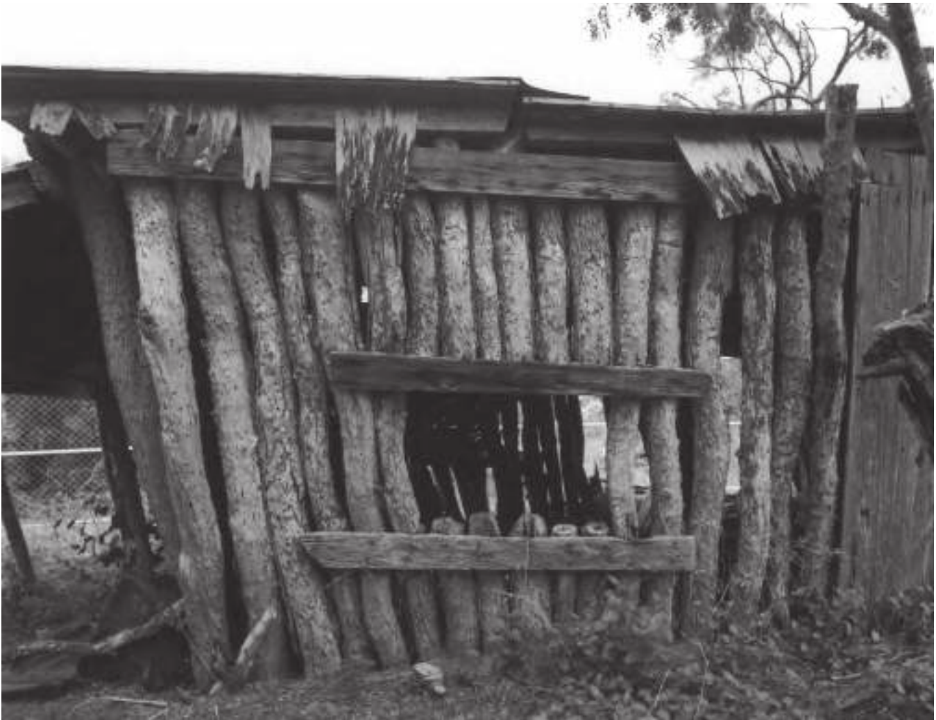
Figure C-7. View of jacal showing window detail and construction elements, looking west (TX-3539-A-5).
