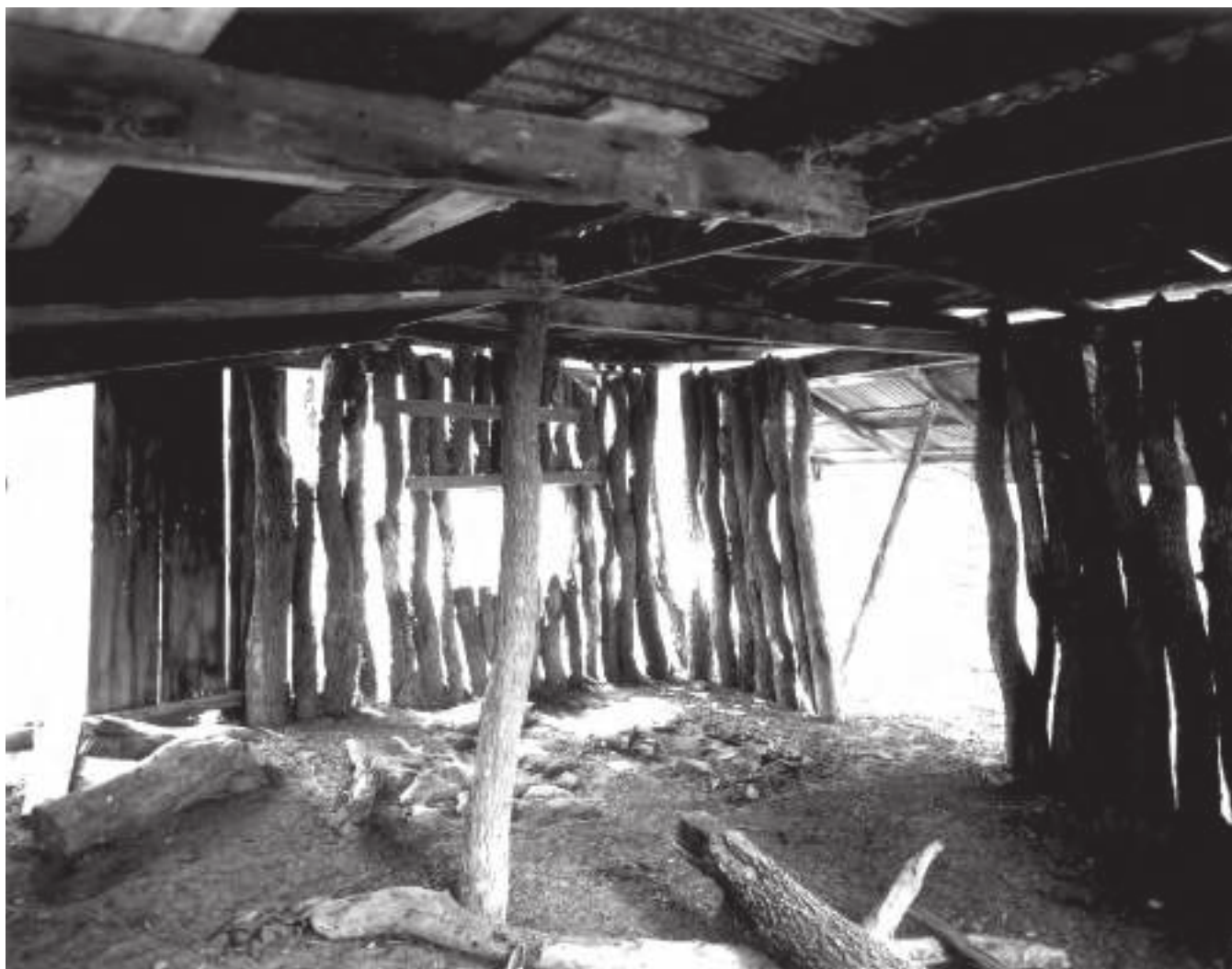
Figure C-13. Interior view of jacal looking southeast to front door and east window (TX-3539-A-11).
