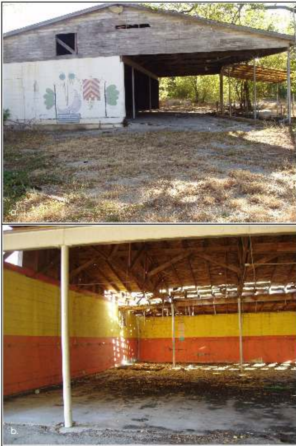
Figure 3-10. Structure 4: a) showing the open roofed side; b) interior of Structure 4, showing poor condition of roof.
