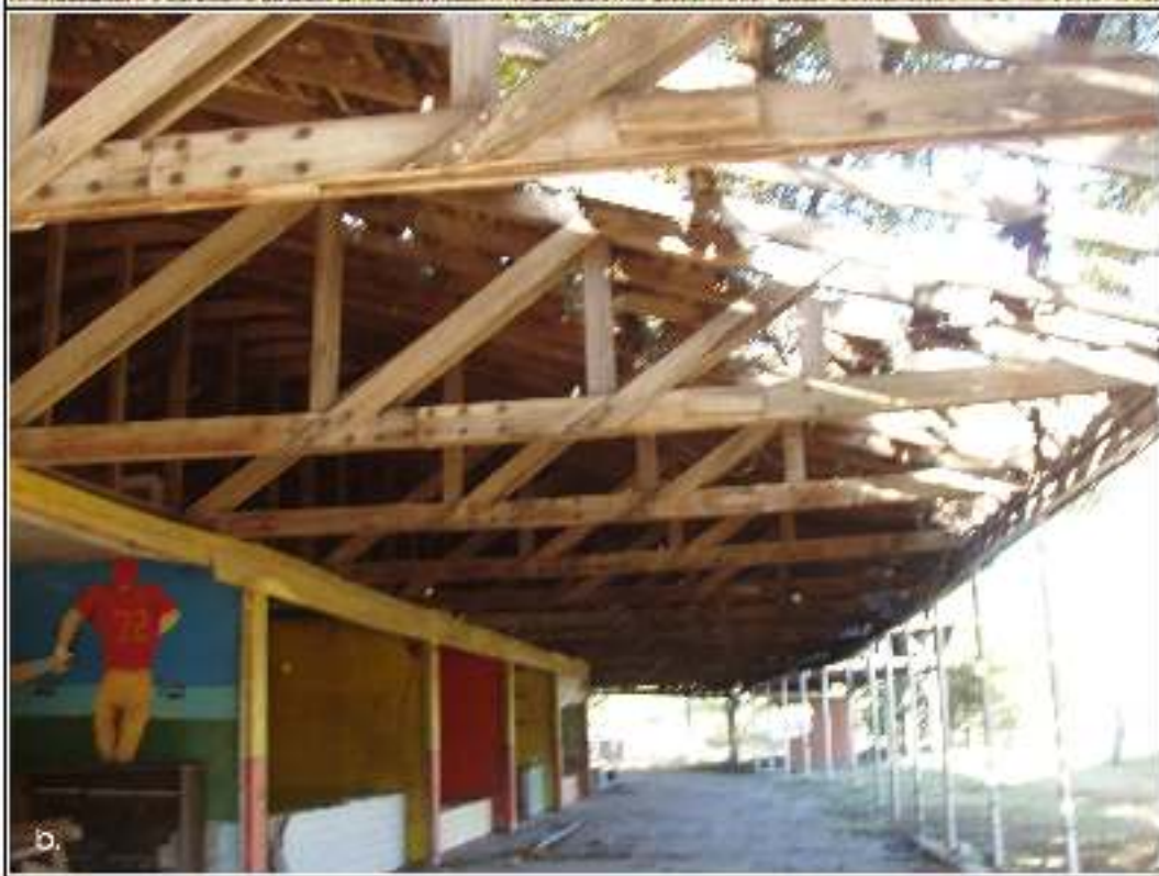
Figure 3-5. View of "the Midway" showing open side with wooden roof above it: a) overview from the east side; b) view of condition of the overhang.
