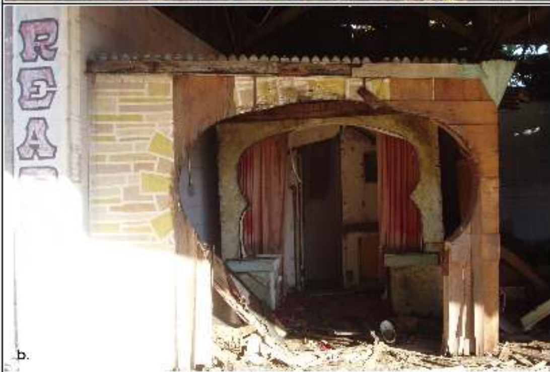
Figure 3-4. Structure 1, showing degree of deterioration: a) view from east b) closer view of the remains of the former-teller's section.
