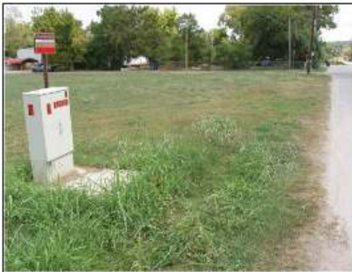
Figure 4-2. East/West course of buried fiber-optic cable along southern boundary of Block 53.
