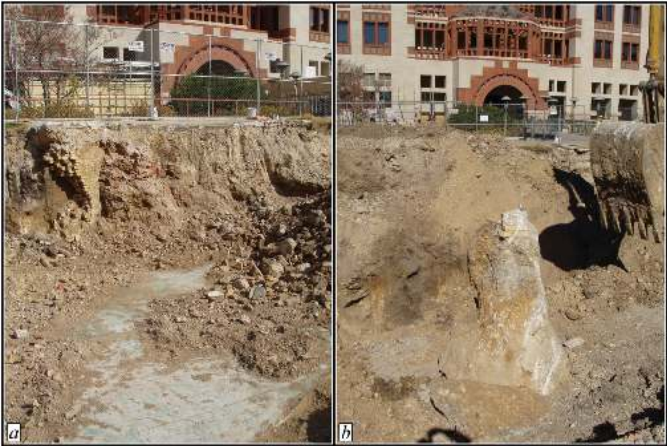
Figure 4-21. a) Evidence of deep impacts to the western portion of the APE (note concrete floor) b) Evidence of deep impacts to western portion of the APE (note the concrete bell-footers).
