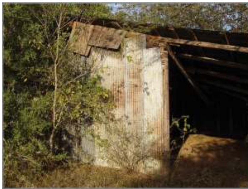
Figure 4-5. Standing metal structure, possibly a cowshed, located in the northwestern portion of the project area.
