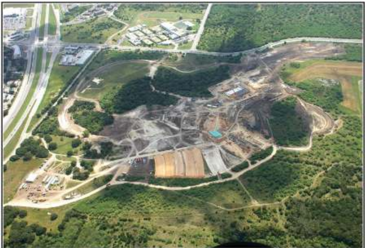
Figure 4-1. Aerial of area showing the amount of disturbance due to construction activities at time of survey.
