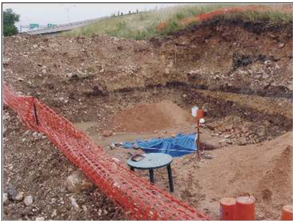
Figure 4-20. Flooding of excavation block during heavy rains.
