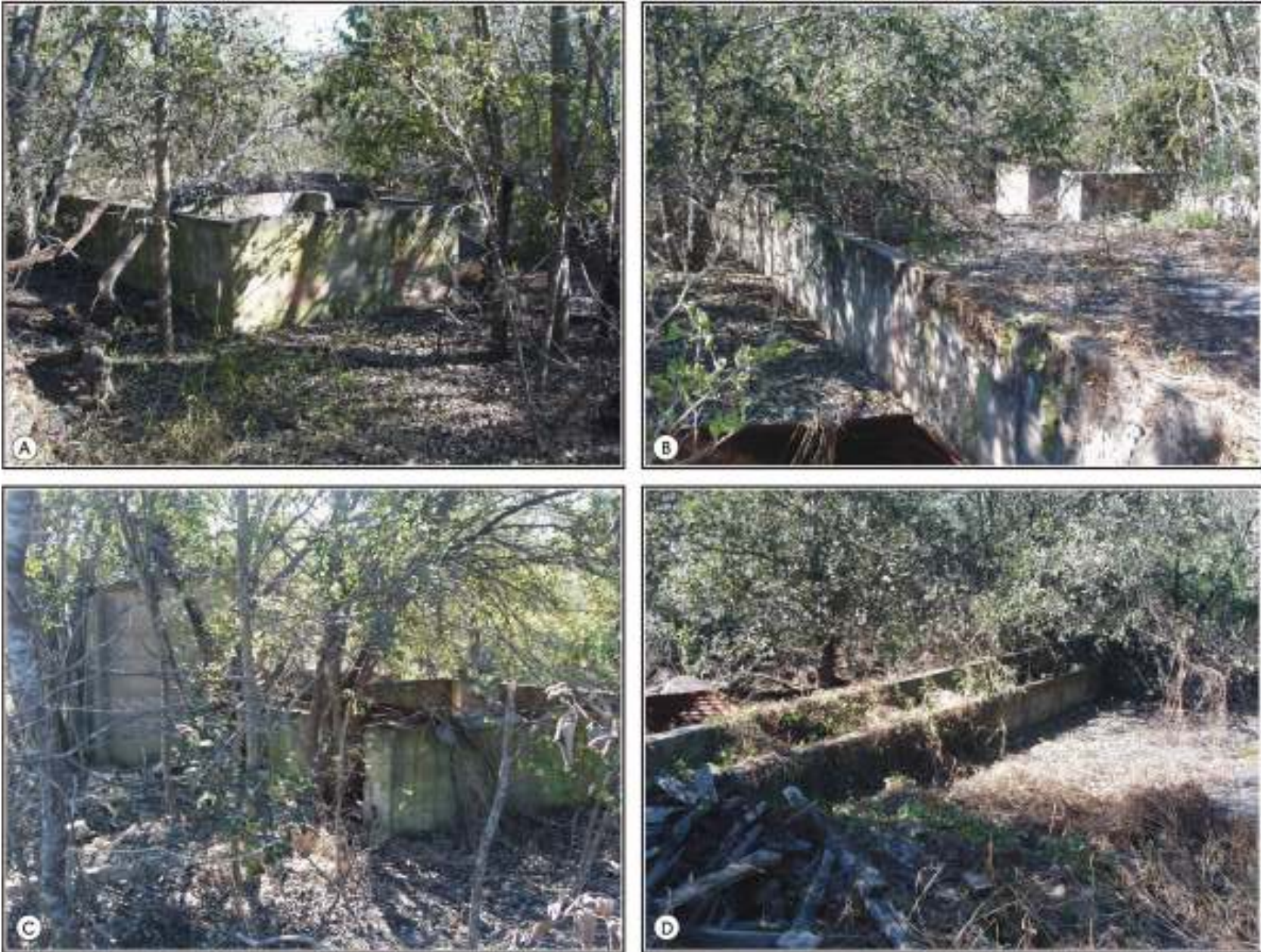
Figure 4-4. Details of concrete structure. Image A shows room 1, the northeast section of the building from the exterior. Image B shows exterior of building from the southwest. Image C shows rooms 3 and 5 from the northeast. Image D is an interior view showing concrete “bins.”
