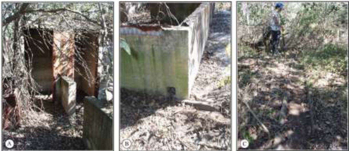
Figure 4-5. Details of concrete structure. Image A shows detail of rooms 3, 4, and 5 from the interior. Image B shows drainage hole from building. Image C shows drainage trough from building.
