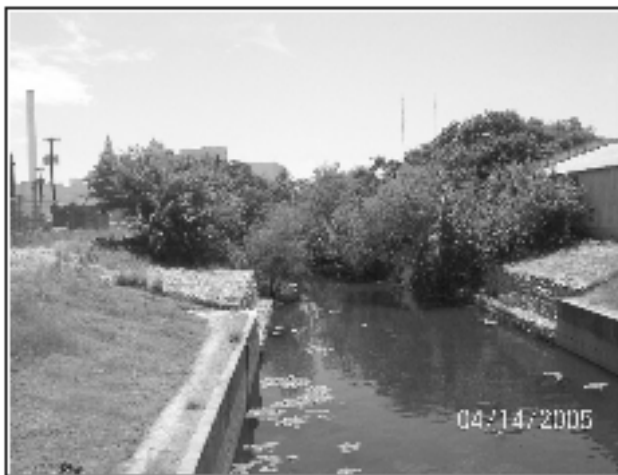
Figure 4-1. Concrete embankments near the northern end of project area, looking south from E. Josephine Street Bridge.
