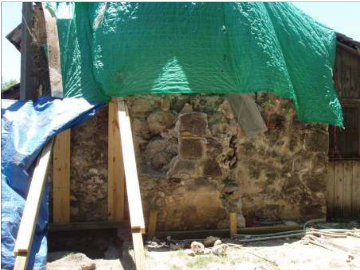
Figure 2. The collapsed chimney and north wall of Room 4.
