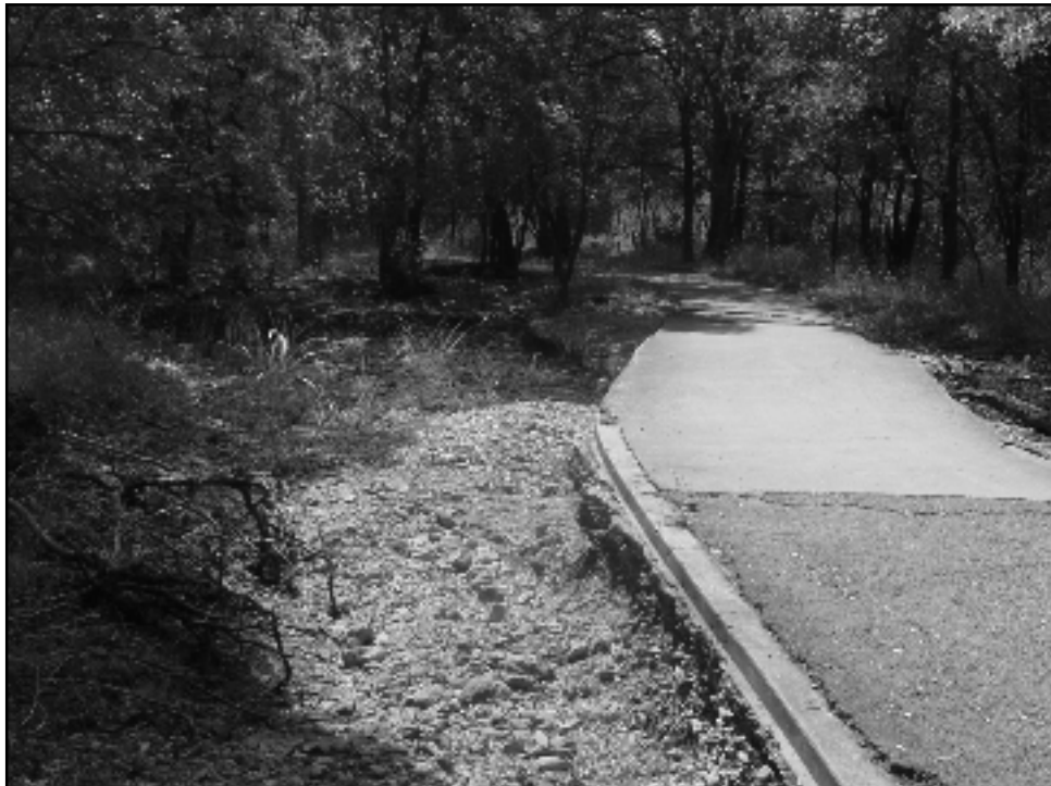
Figure 1-9. Low-water crossing of Lorenz Creek in Area 7. Note erosion at base of sidewalk.
