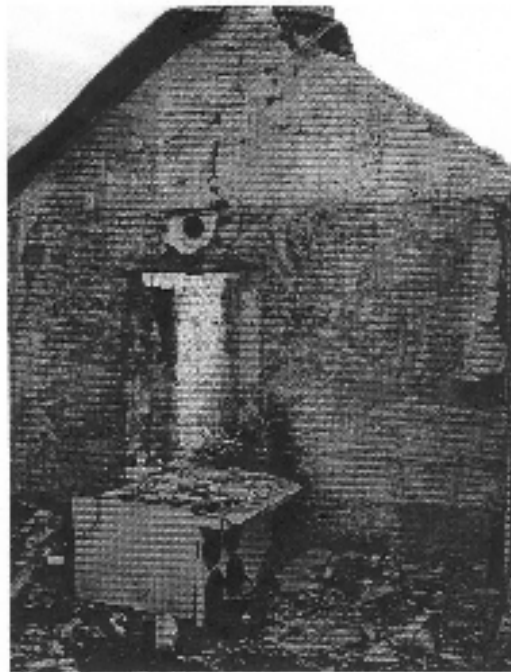
PHOTO 4: Additional view of structure after the fire.
