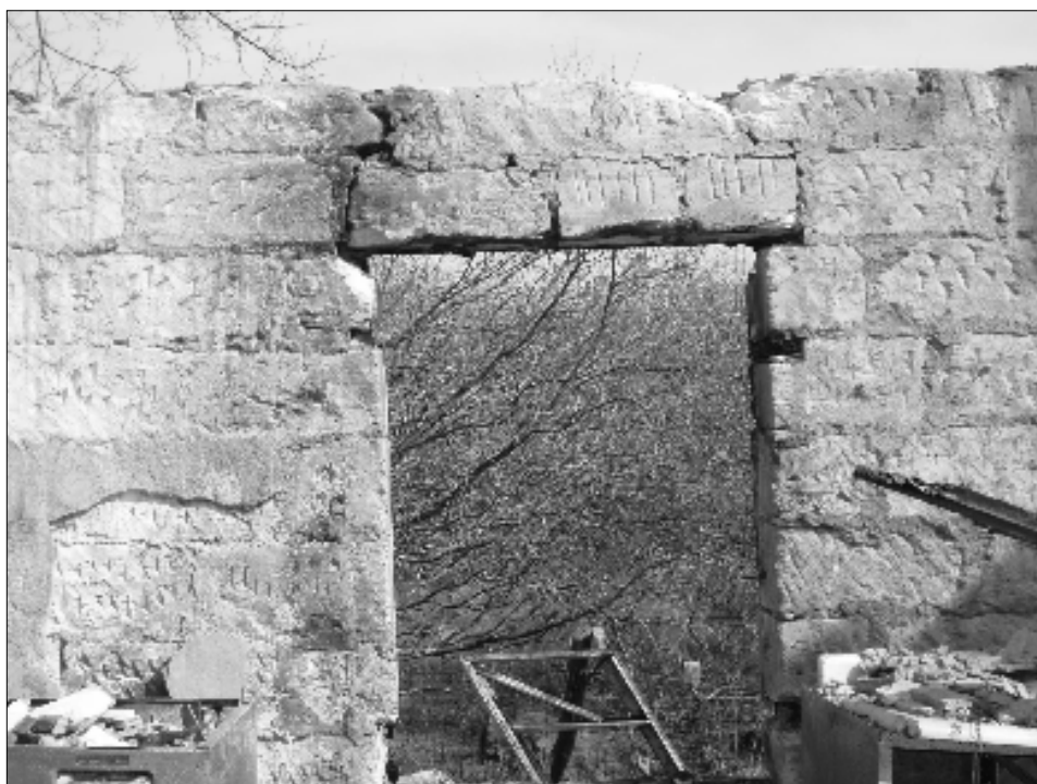
Figure 48. Addition 3 of homestead with no keystones present and chisel marks on the limestone blocks (facing north).
