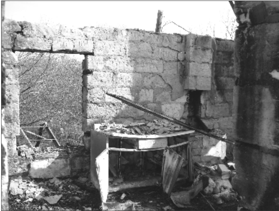
Figure 44. Hearth in north wall of Addition 3. Also note north wall window and stonework detail.
