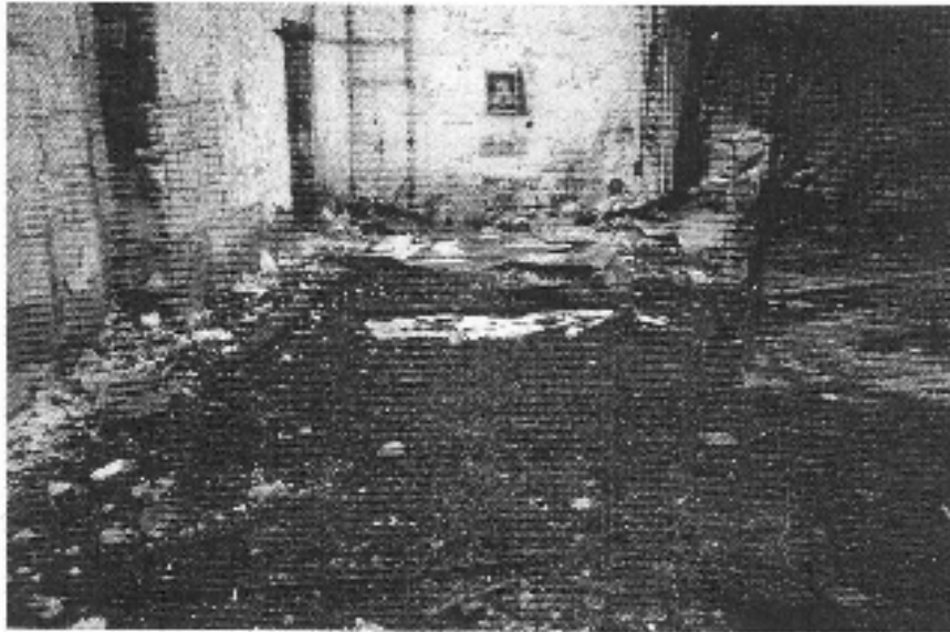
PHOTO 9: View of asbestos containing debris present within the footprint of the structure after the fire.
