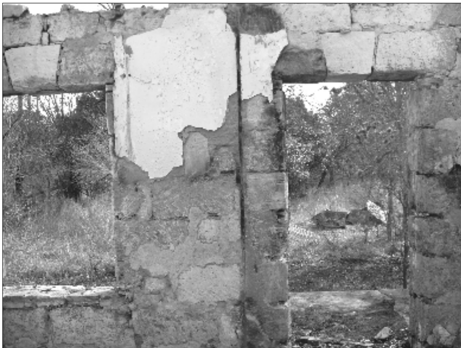
Figure 41. Inside of original portion of homestead employing keystone above the window and doorway (facing west).
