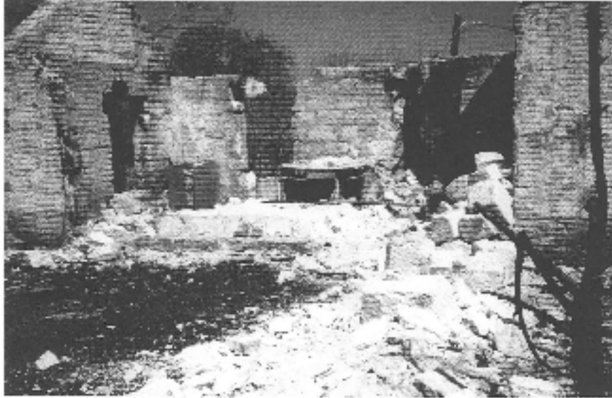
PHOTO 13: View of same wall in Photo 12 on March 11, 2005. Also shows west wall remaining as a free standing wall.
