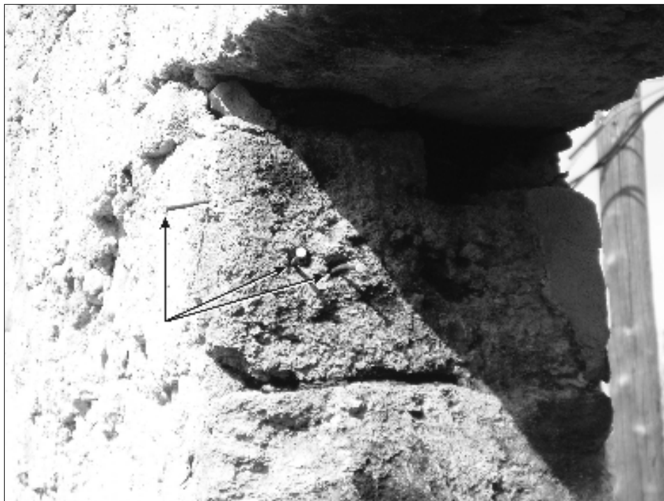
Figure 47. Wire nails that originally supported wood framing around the west doorway of Addition 2.
