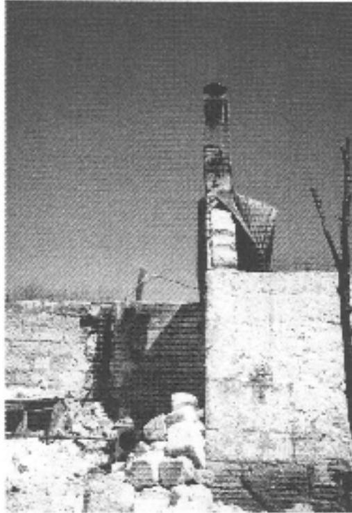
PHOTO 17: View of center wall with chimney now without the support of the south wall.
