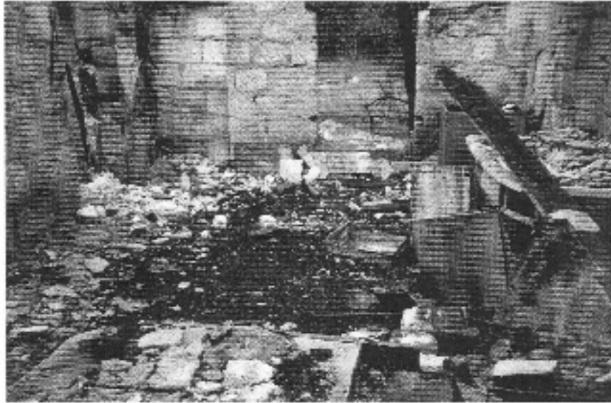
PHOTO 11: Additional view of asbestos containing debris present.
