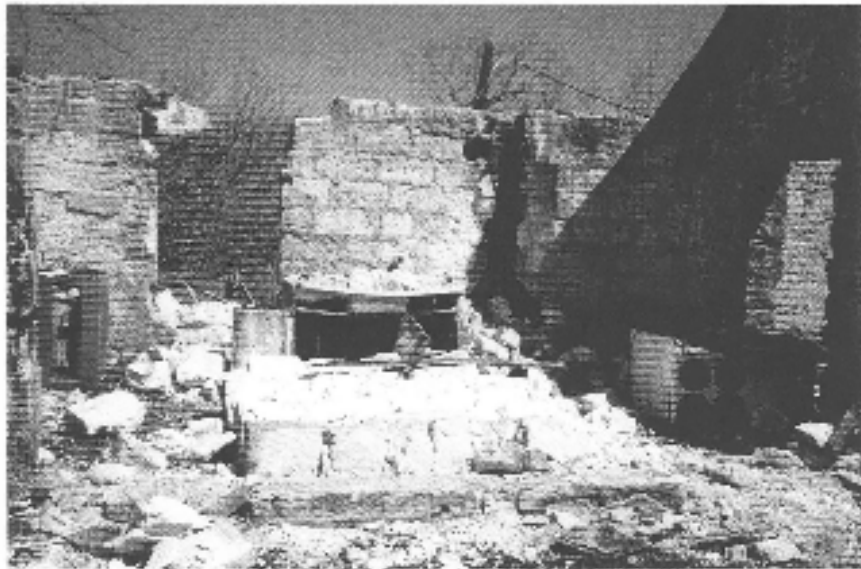
PHOTO 14: View of south wall section that collapsed inward.
