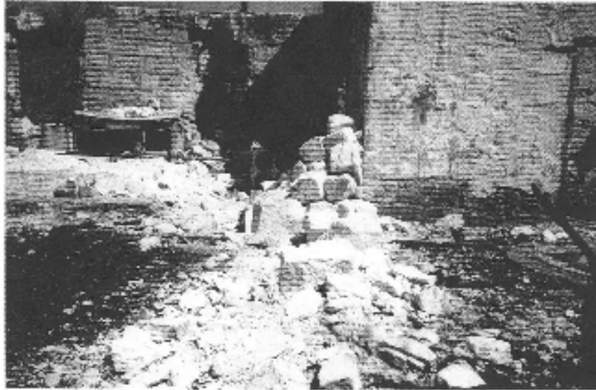
PHOTO 15: View depicting the extent of south wall outwards.
