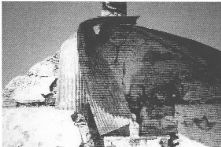
PHOTO 18: View of chimney base that has been weakened.
