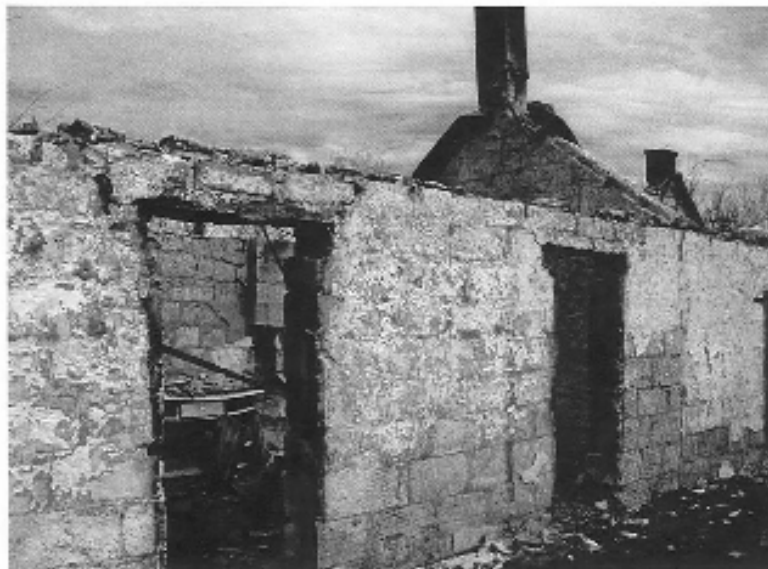
PHOTO 2: Additional view of structure after the fire.
