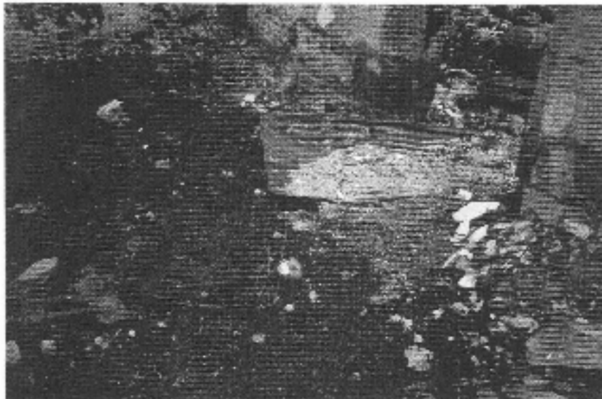
PHOTO 10: Additional view of asbestos containing debris present within the footprint of the structure.
