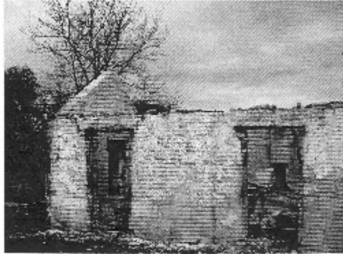
PHOTO 3: Additional view of structure after the fire.
