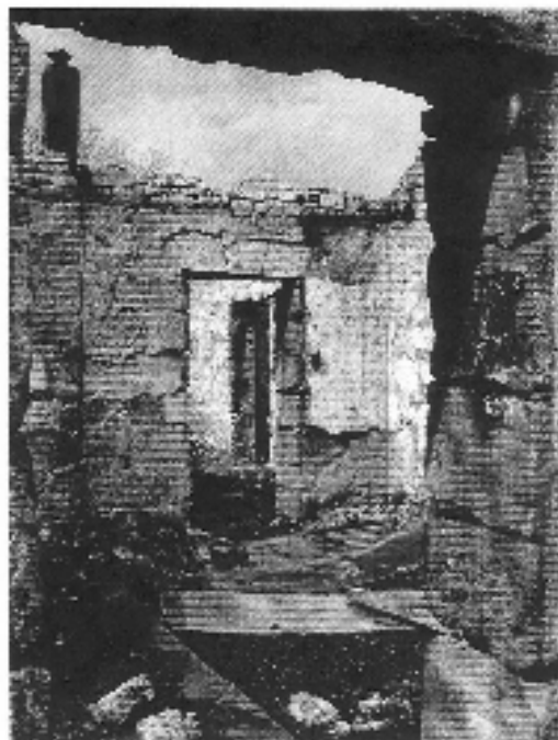
PHOTO 6: Additional view of structure after the fire.
