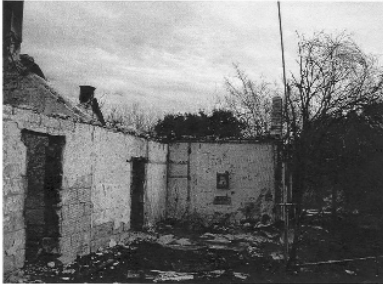
PHOTO 1: View of structure after the fire in January 2005.
