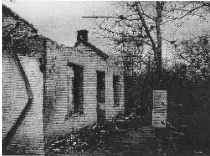
PHOTO 5: Additional view of structure after the fire.
