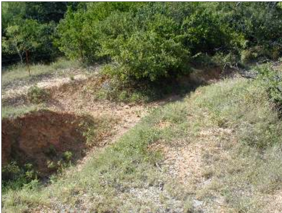
Figure 4-24. Photo of erosion at 41BX1580.
