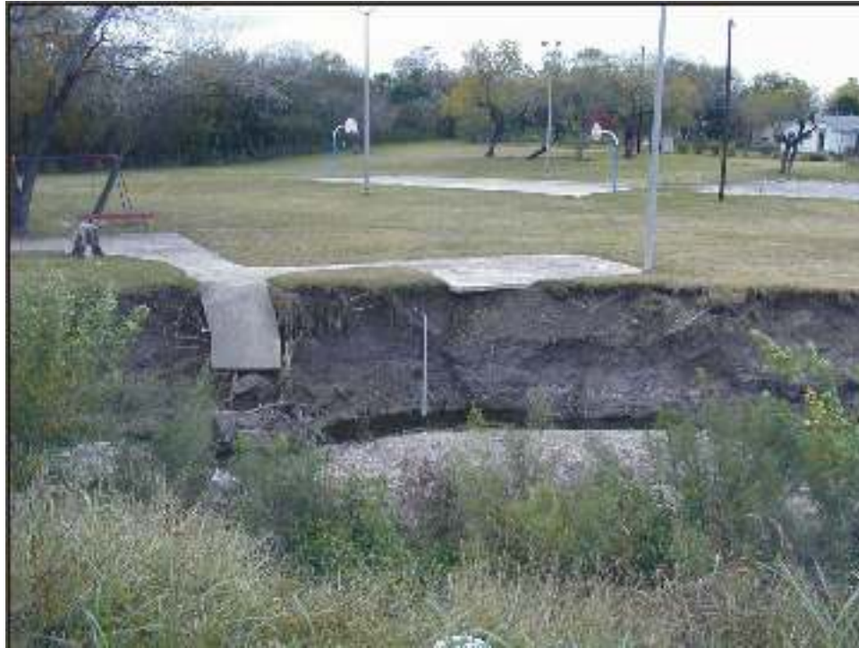
Figure 10. Disturbances along west bank of Salado Creek at Crossing 1.
