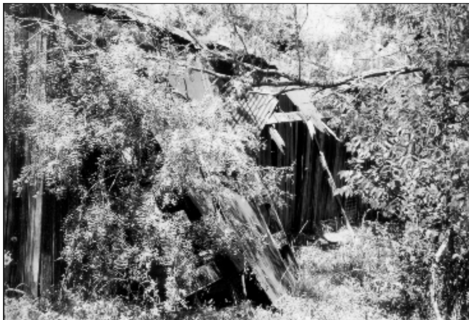
Figure 5-51. Collapsed third room of tenant house, 41BX661.
