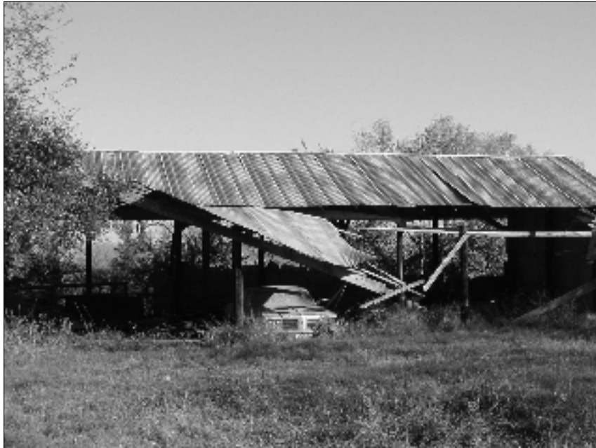
Figure 5-14. Partially collapsed barn/stall, 41BX681.
