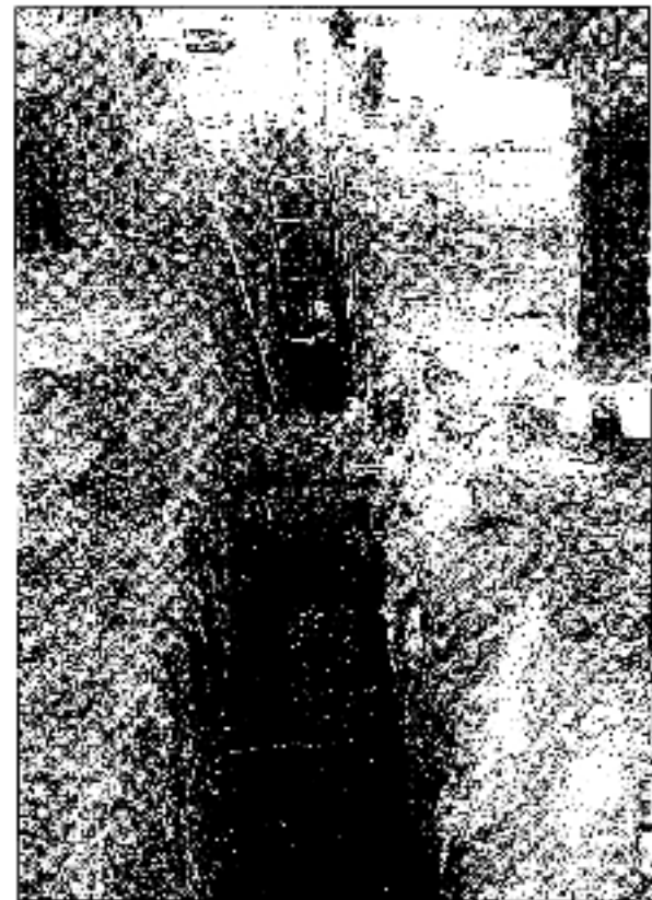
Figure 5-7. Photo showing trench for Drainage System A storm sewer passing under reinforced concrete pipe carrying the Espada Acequia.
