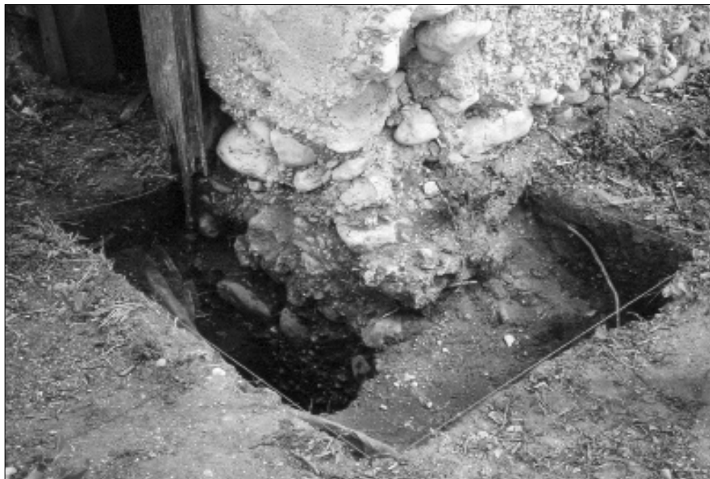
Figure 9. Base of wall and footing exposed in Unit 3 adjacent the southwest corner of the structure.
