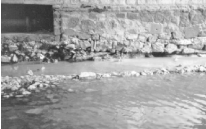
Figure 9. 41BX1370 - Artifact deposit beneath pilot channel retaining wall.
