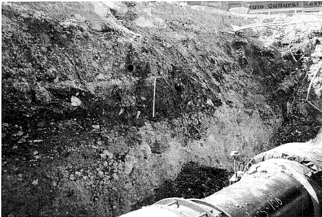
Figure 17. Acequia Feature 11 . Note relationship of the clay pipe (left of measuring tape above) to the acequia deposit in the skematic profile below.
